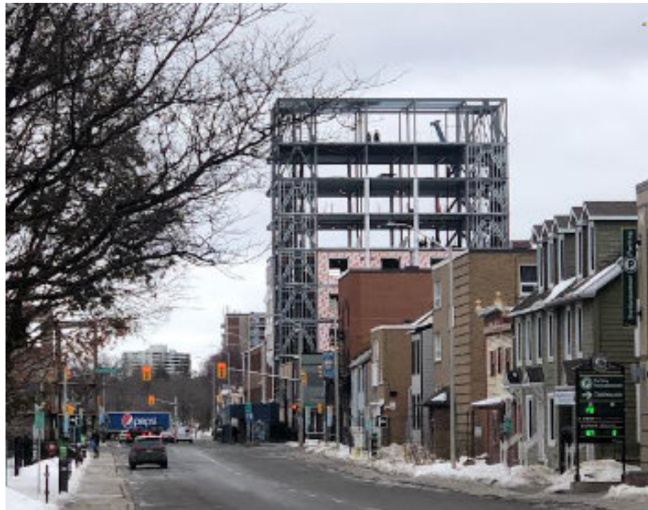
Shepherds of Good Hope building under construction on Murray Street (Photo: Allen Brown)
